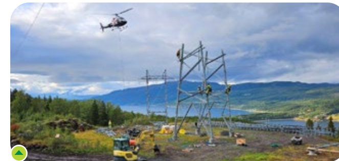
132kV S-C Transmission Line in Norway
