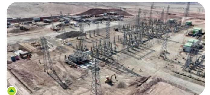
220/110 KV AIS Substation in Chile
