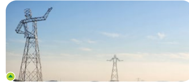
500 kV HVDC 200 km Transmission Line from Tajikistan Border to Afghanistan
