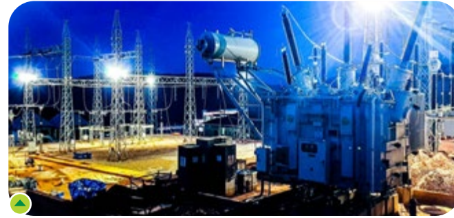
220-132 kV Substation in Burundi
