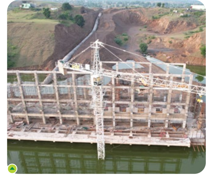
24 MLD Lahchura Water Supply Scheme in Uttar Pradesh
