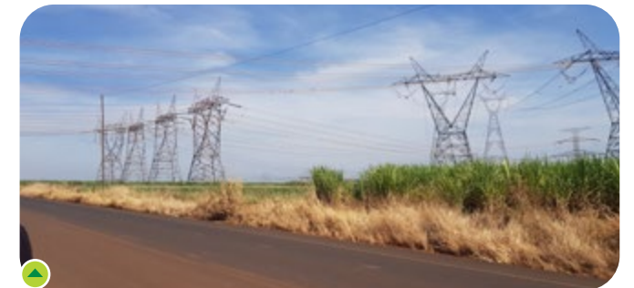
500 kV Double Circuit line in Brazil
