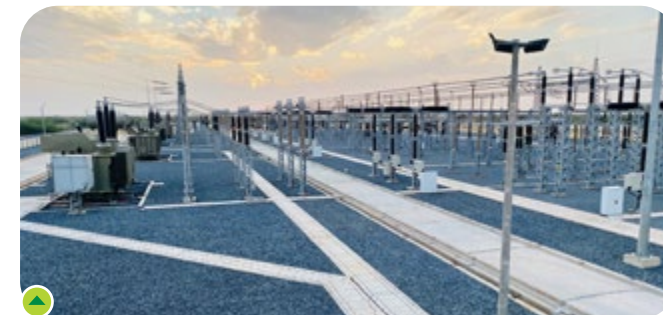
225/30 KV Substation in Senegal
