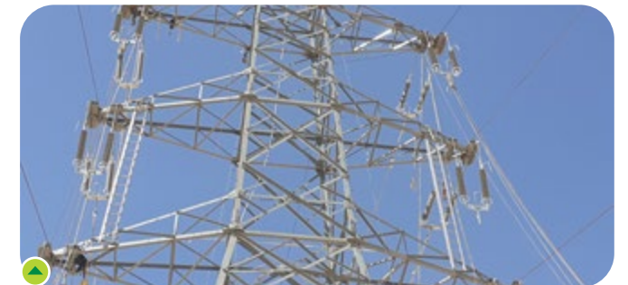
225 kV Double Circuit line in Mauritania
