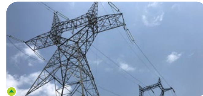
225 kV Single Circuit line in Cameroon
