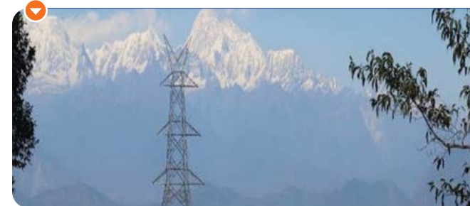
Nepal Koshi Corridor 400 kV D/C Transmission Line
