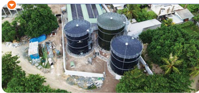
Construction of water and sewerage facilities including RTP and Admin buildings across 10 Maldivian islands.
