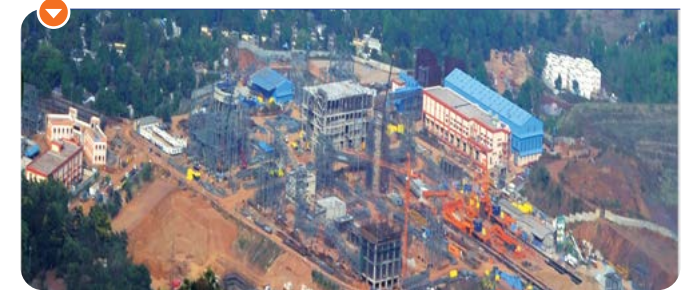
Iron Ore Beneficial Plant, Bachel
